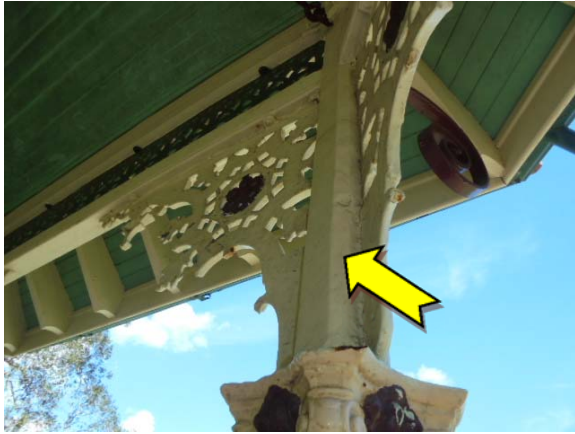
Photo 1. Exterior, throughout, railing – suspected lead-containing white upper paint system.
