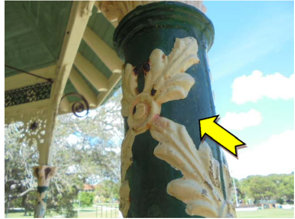
Photo 2. Exterior, throughout, support rails – suspected lead-containing green upper paint system.
